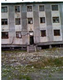
Figure 2. Deformation of structure from possible loss in bearing capacity of the frozen ground
